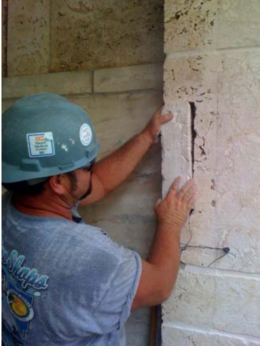
A mason works on repairing damaged oolitic limestone walls on historic building.
